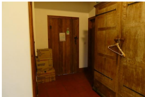
Approach to accessible WC door is obstructed by cupboard and has small high sign
