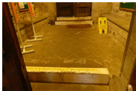
View from inner double doors towards two steps up to outer double doors
