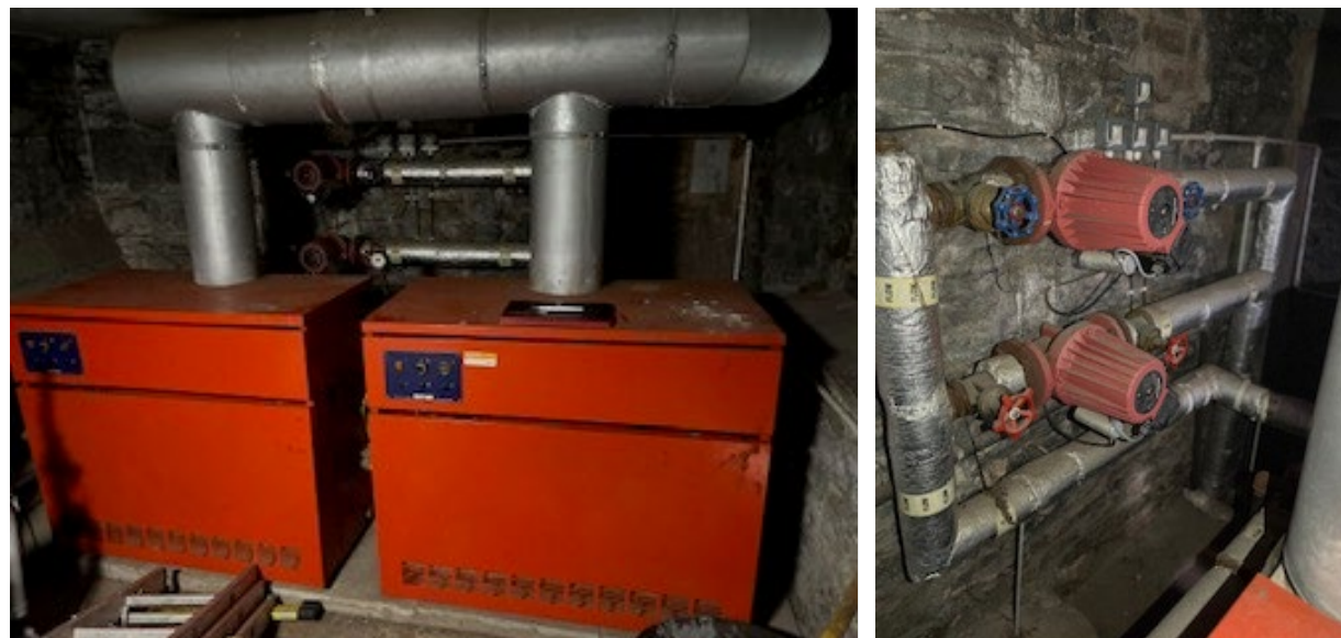
Figure 8: Heating for the Cathedral provided by two 325kW boilers.
