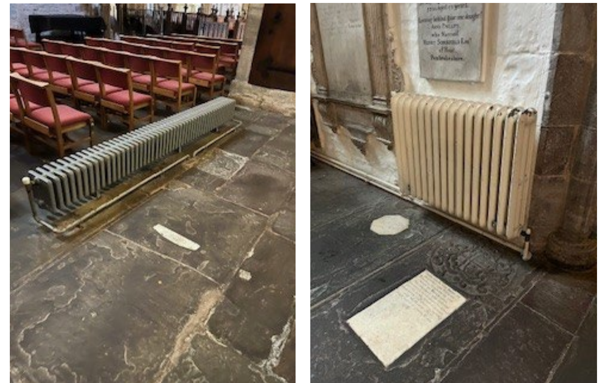
Figure 9: Cathedral heat emitters & distribution system.
